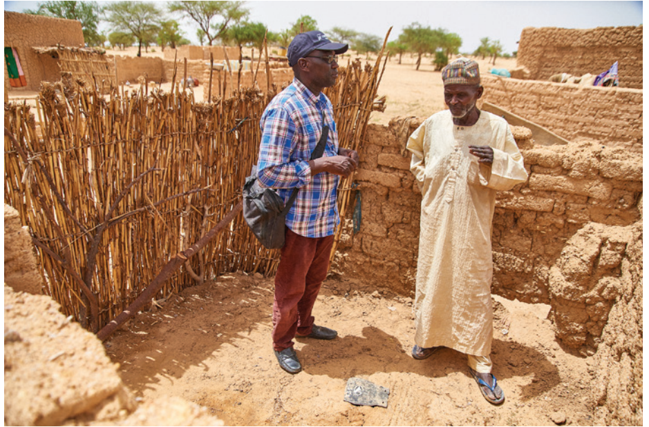
A sanitation worker and village chief discuss the construction of a latrine at the chief's home in the Zinder region of Niger. Last year, The Carter Center assisted in the construction of more than 10,000 latrines in Niger and Mali.
